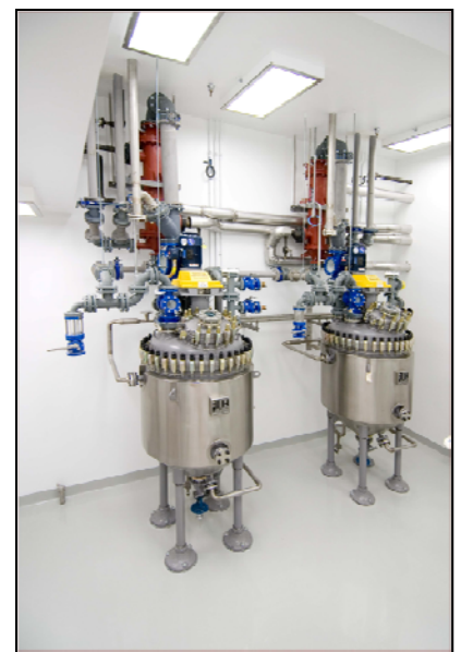
TANTALUM PHARMACEUTICAL CONDENSERS INSTALLED WITH GLASS LINED STEEL REACTORS
